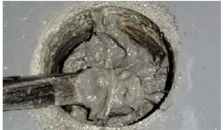
Water below the surface is eating away at the existing epoxy floor. This paste of decomposing epoxy was hiding underneath.
