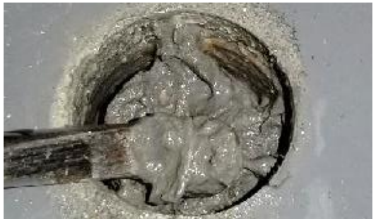
Water below the surface is eating away at the existing epoxy floor. This paste of decomposing epoxy was hiding underneath.
